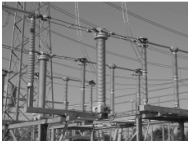
Figure 11-42. 362 kV Optical Metering Units at Substation.
