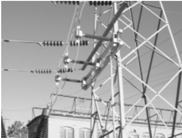
Figure 11-41. 72 kV Magneto-Optic Current Transducers at Substation.
